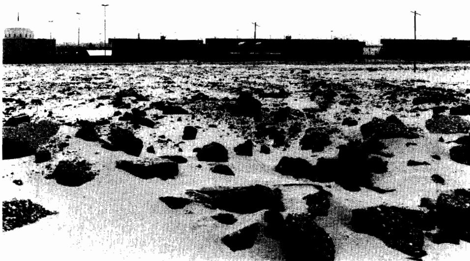
Fig. 6. Used asphalt scattered of over the sand surface to stabilize the local sand.
